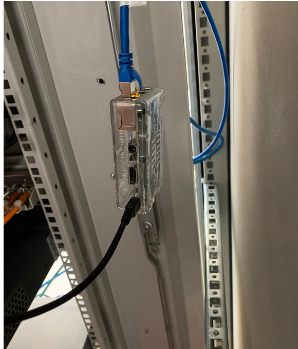
Figure 5.1: The Raspberry Pi from the experiment placed in the back of a network distribution cabinet. On the left side, some network devices are stacked. It is placed behind a cover, so it is not visible when looking through the glass door or even when opening it.
